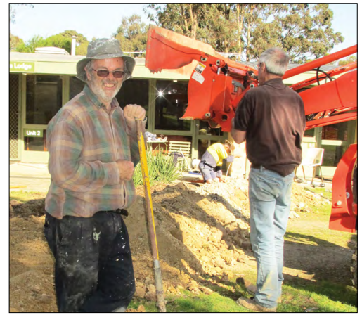
Peter Dedrick on shovel, Peter Gillespie adjusting the backhoe and Peter Dunstan in the trench
